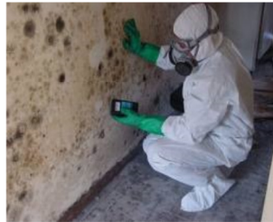
Large amount of mold
