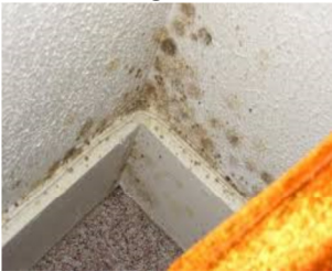
Small amount of mold
